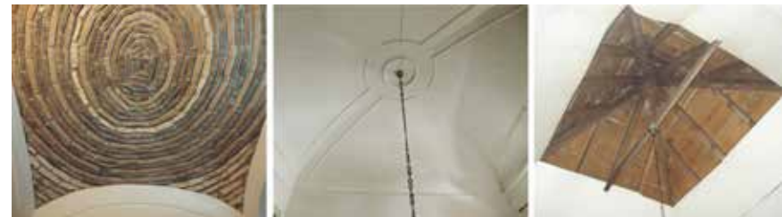
14. Photography of the interior of the roof of the main room casa de fora of houses in Fuzeta: sail vault, dominical vault and pitched roof. (Author's photos)
